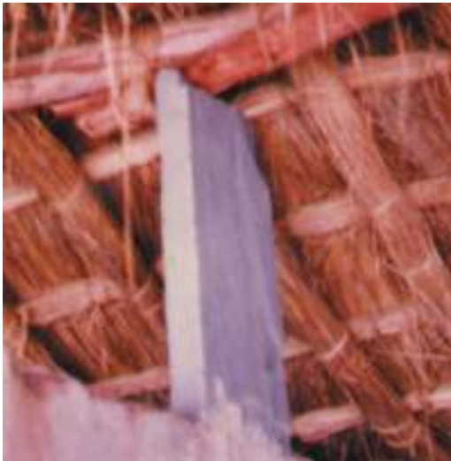
Digantar school : Roof construction detail showing Vertical Stone Patti, Wooden Ballis and Thatch Roof
