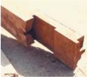
The dismantled beam
